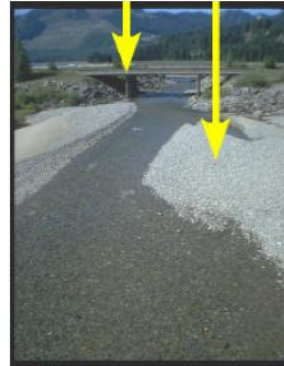
Poor Range (arrows emphasizing large-scale channel alterations)
